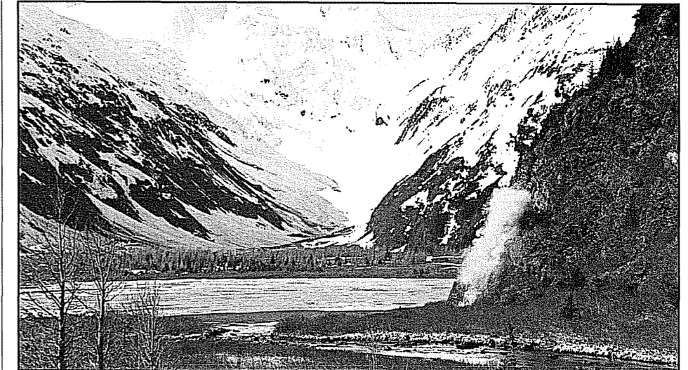
With Portage Lake in the background, the ceremonial blast for the Whittier road took place in Bear Valley in early May.
