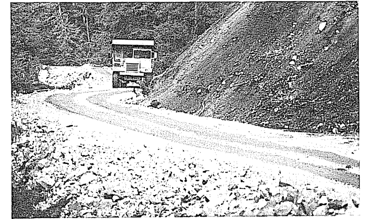
The 14-foot wide Quartz Hill Access Road is now open to heavy truck traffic.
