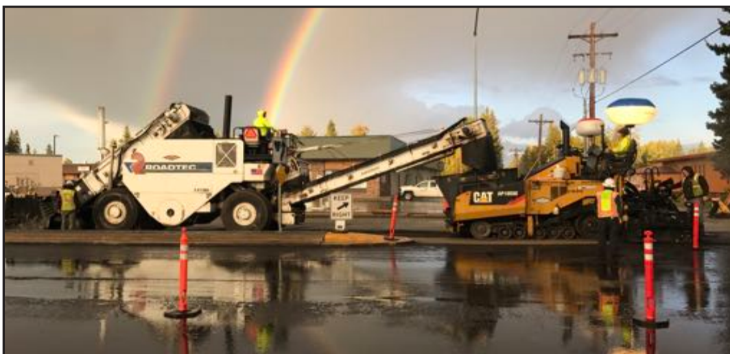
Farmers Loop Resurfacing and Farmers Loop Signal Interconnect – Colaska, Inc. – Exclusive Paving
