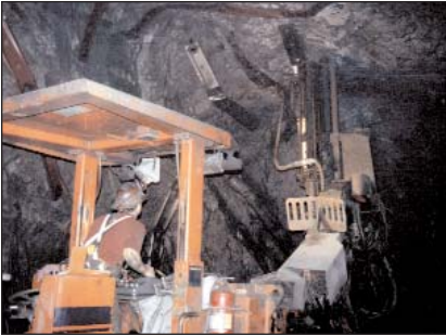
A miner prepares the work area for drilling and blasting inside the Greens Creek Mine. The underground mine has miles of tunnels extending more than 1,000 feet below the surface. After blasting the ore is hauled to the mill where it is processed.
