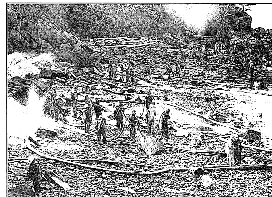
Exxon's shoreline cleanup operations are accelerating. Cleanup crews are shown here at McPherson Bay on Naked Island flushing the oil from the shoreline rocks and recovering it with booms and skimmers. Over 70 vessels and 5,000 people will be involved in cleanup operations this summer. photo by Frank Flavin
