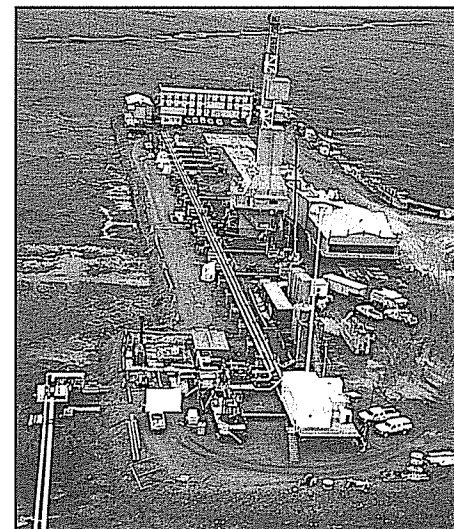
A Doyon drilling rig operates on one of Tarn's two gravel pads.
