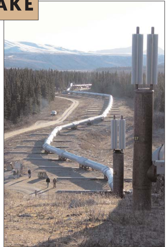
Crews inspect support structures for the pipeline where it crosses the Denali fault. In this location, the supports for the pipeline are built directly on the ground, allowing for intentional movement in a big quake.
