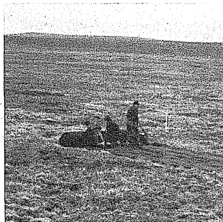
Workers lay geotextile fabric out on the tundra as work begins on the Red Dog haul road.
