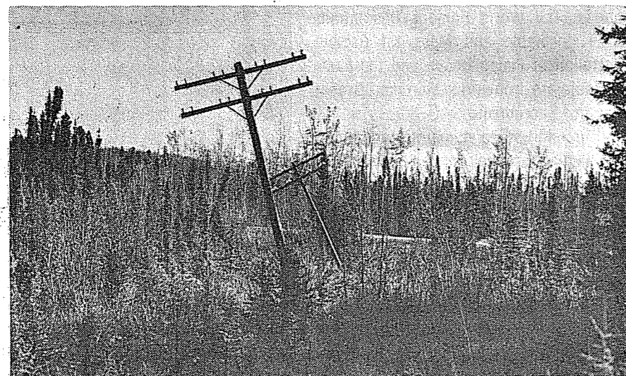
Tilted utility poles in moist terrain is a common sight in Alaska.
