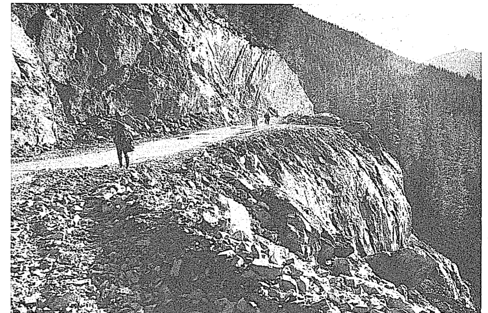
The access and bulk sampling road from tidewater to the U.S. Borax Quartz Hill molybdenum deposit was one of the most heavily regulated and monitored road construction projects ever undertaken in Alaska. Environmental permits in 20 different categories from nine separate agencies were needed before the ten mile road was completed in 1983.
