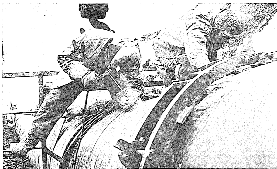
Construction of a gas pipeline across Alaska will result in thousands of new jobs for Alaskans. These pipeline welders "tied-in" the final weld for the Thompson Pass section of the oil pipeline in 1976.
